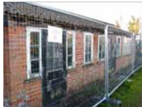
Brick structures on the north side of the walled garden are in poor condition
