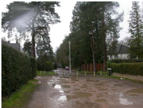
Plate 39: Pot holes in the lanes serving Church Street cause water to pool in some places making pedestrian access difficult. These have recently been repaired
