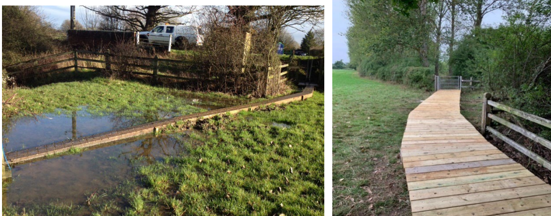
Figure 25 Before and after pictures of improvements. The new section of boardwalk, which is pictured to the right, will receive grip strips to improve its usability.
